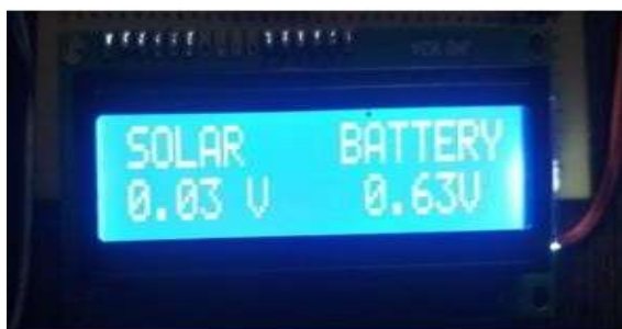
Fig1. LCD displaying voltage in solar panel and battery.
