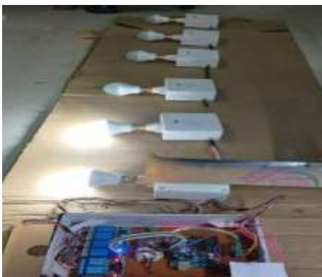
Figure 6. Operation Phase 2 of street light automation
