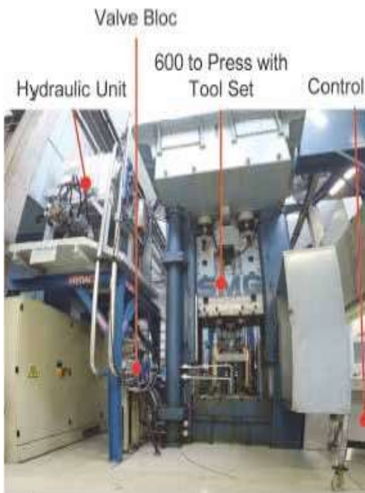
Fig.5. Hydraulic unit with valve bloc, hydraulic press with and control unit
